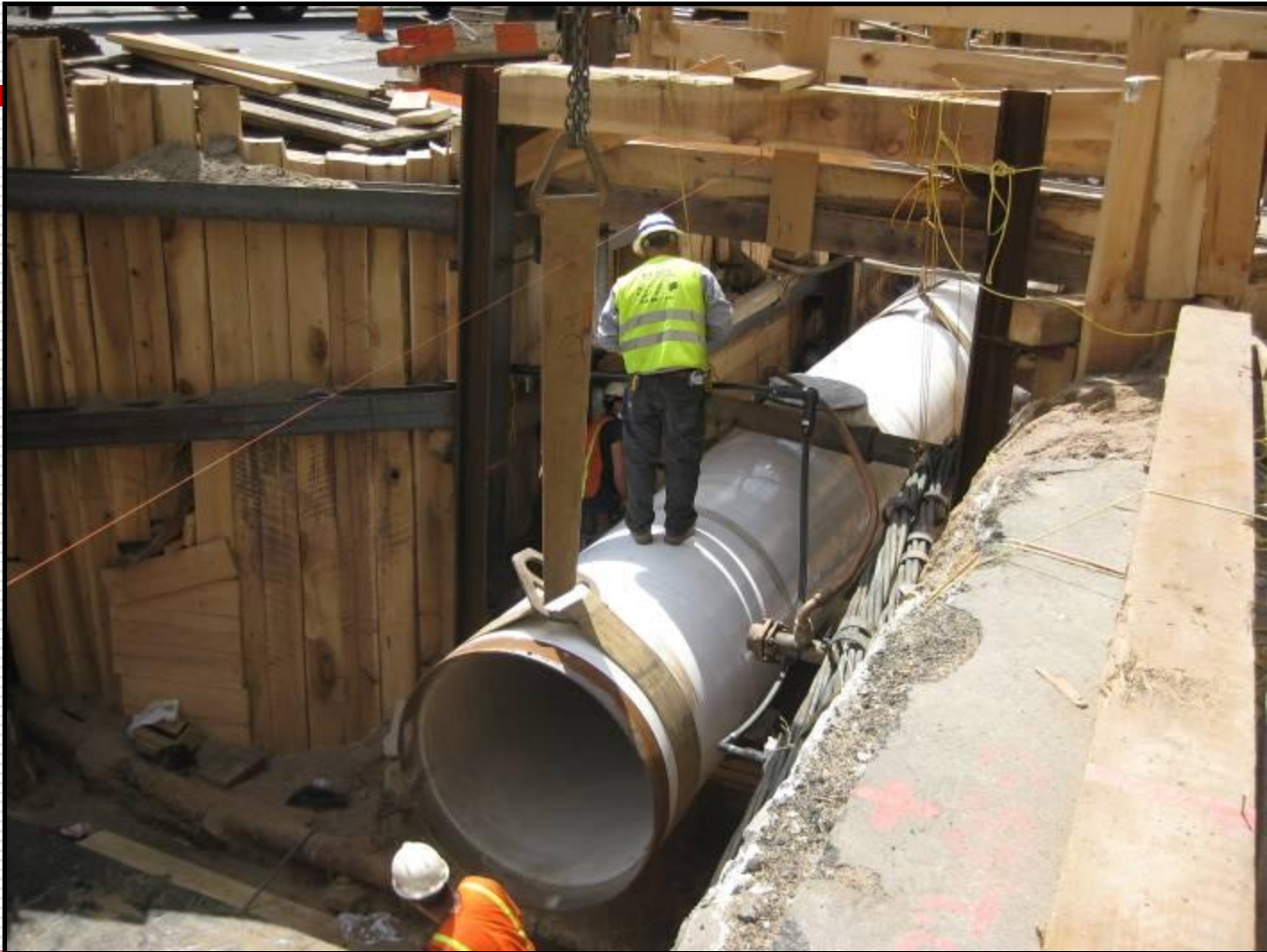
INSTALLATION OF TRUNK WATER MAINS IN W.48 th STREET Project ID: MED599
